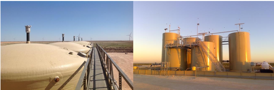
Standpipe with vacuum/pressure relief valve
