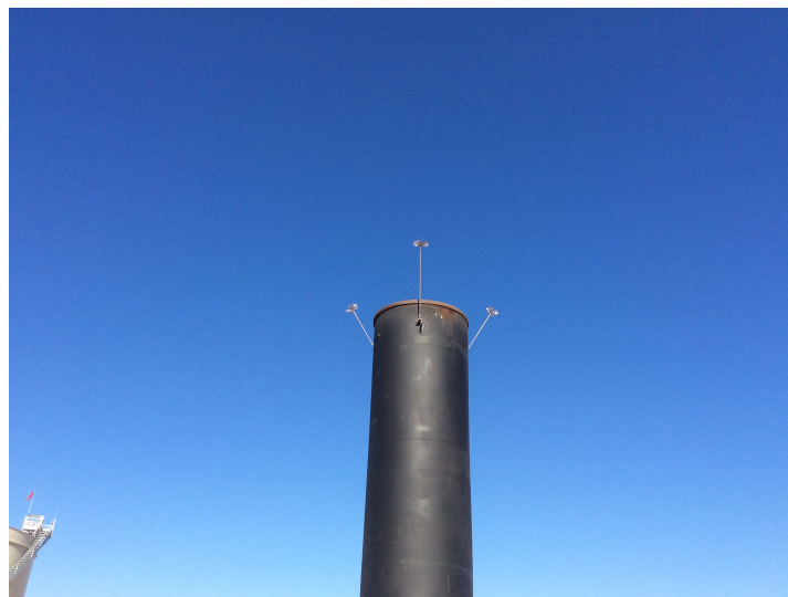
Air Terminals on Exhaust Stack
