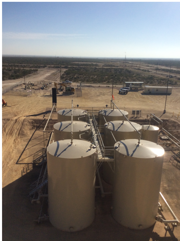
Structural Lightning Protection on Tank Battery
