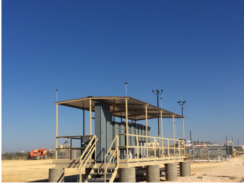
Structural Lightning Protection on MCC Shelter
