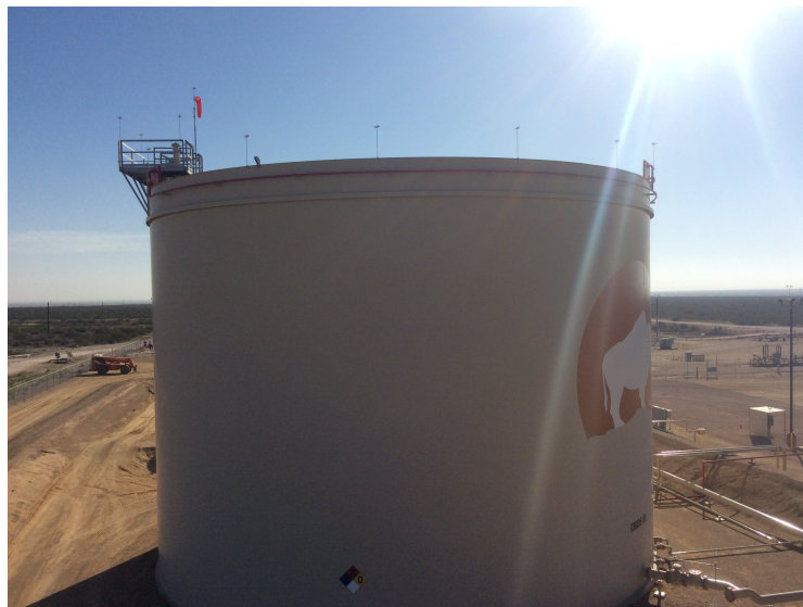
Structural Lightning Protection on EFR Tank
