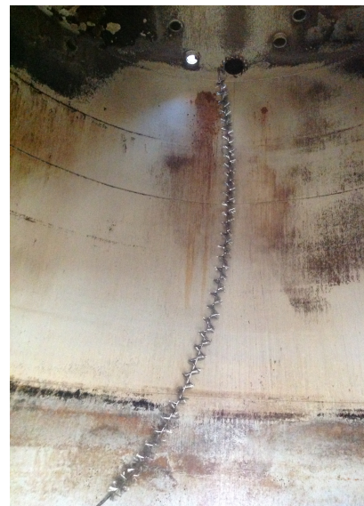
ITSD inside a production tank
