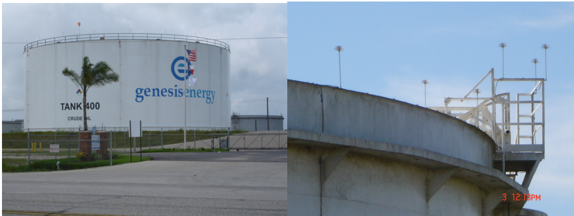
Streamer delaying air terminals on storage tanks
