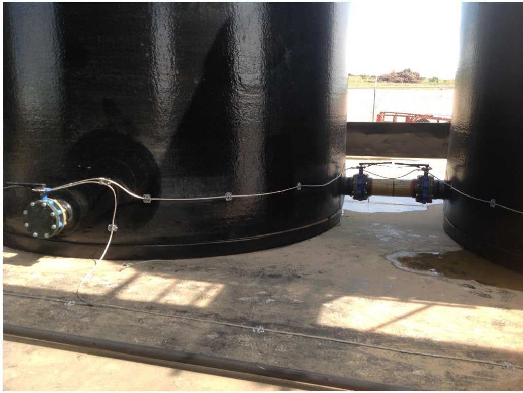
tank base and valve bonding
