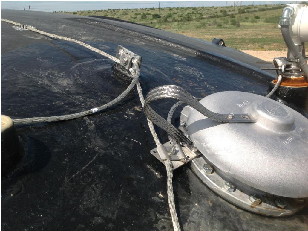
tank-top piping, thief hatch, and walkway bonding
