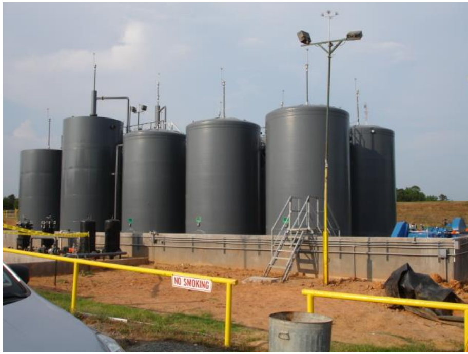
air terminals on tank battery
