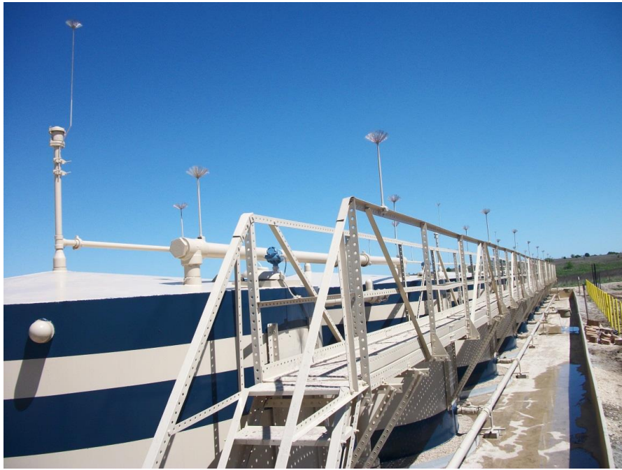
streamer-delaying air terminals on handrail, piping and Enardo valve
